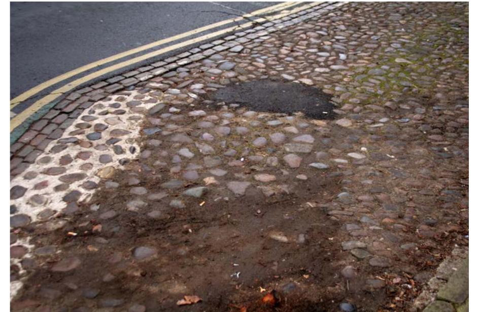
Cobbles on Blossom Street with contrasting reinstatement (white cement) and repair (asphalt) resulting in a significant visual detractor on this historic gateway street. The spacing of reinstated cobbles is also poor.
