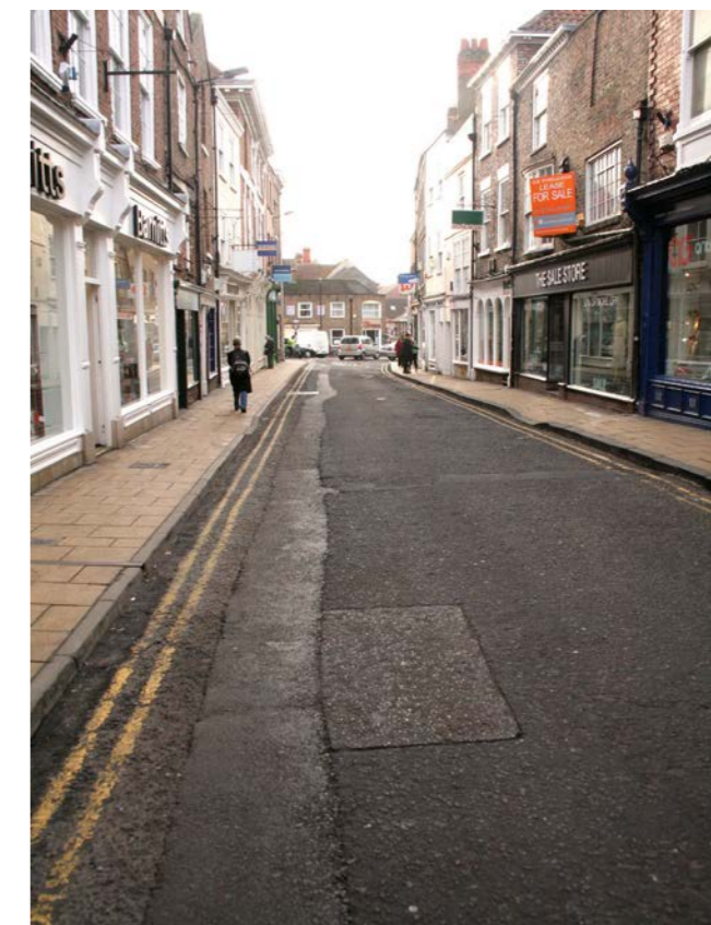
Colliergate with narrow footways badly surfaced in small square pre-cast Saxon flagstones and a poor quality carriageway surface
