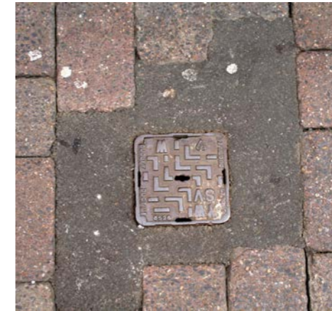
An extremely poor example of repair work by utility contractors using cement rather than the original brick paviours
