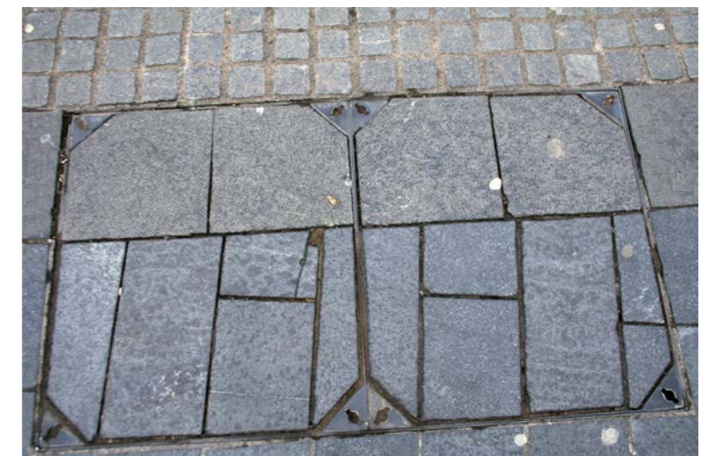
A poor example from Sheffield where more than one material has been used to infill the inspection cover
