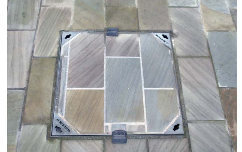
An excellently designed and laid utility inspection cover in Doncaster's cultural quarter. Note the neat jointing.
