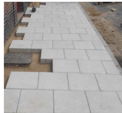
Grey Saxon paving in the process of being laid on Priory Street as a stretcher bond
