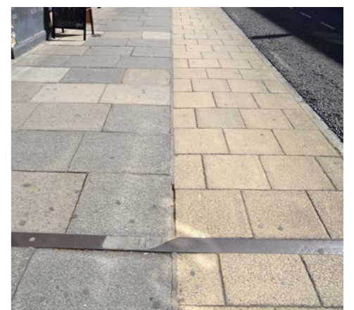
Two different materials used on Micklegate when the pavement was widened, resulting in an unattractive and uncoordinated footway
