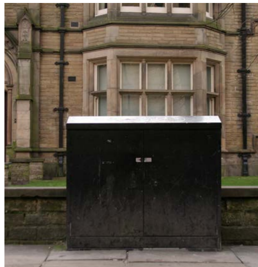
Street cabinet in gloss black, positioned against the pavement back edge on Duncombe Place. Well-positioned but in a challenging location
