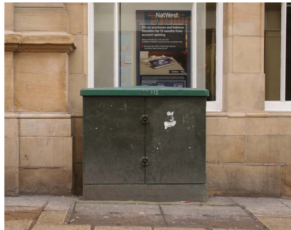
Green cabinet contrasting poorly with warm Magnesian limestone on Market Street in the centre of the footstreets. Gloss black would improve this although relocation would be preferable, where technology changes.
