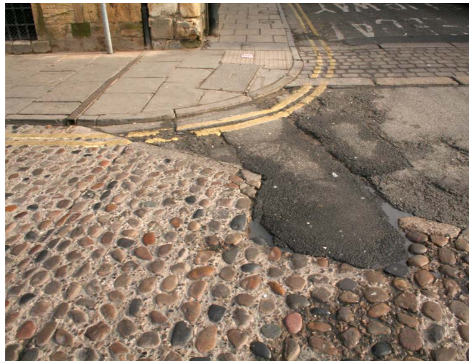
An awful utility company reinstatement of a historic cobbled surface at King's Staith
