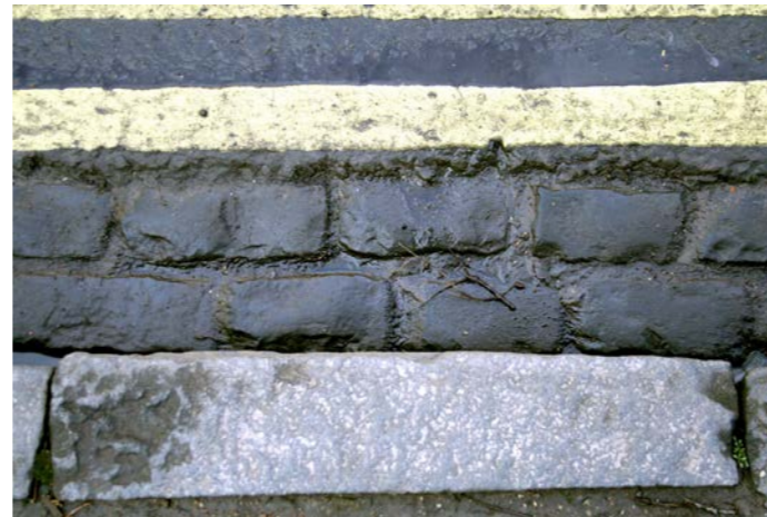
Traditional brick drainage channel in situ parallel to a granite kerb adding interest to the carriageway.
