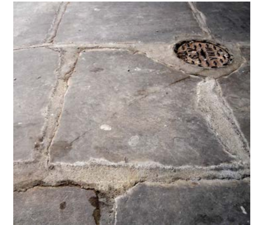
Wide joints in riven English Pennine sandstone poorly pointed with cement mortar
